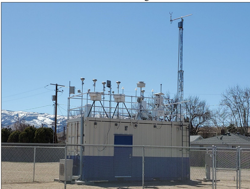
Figure 8 Reno4 Monitoring Station
