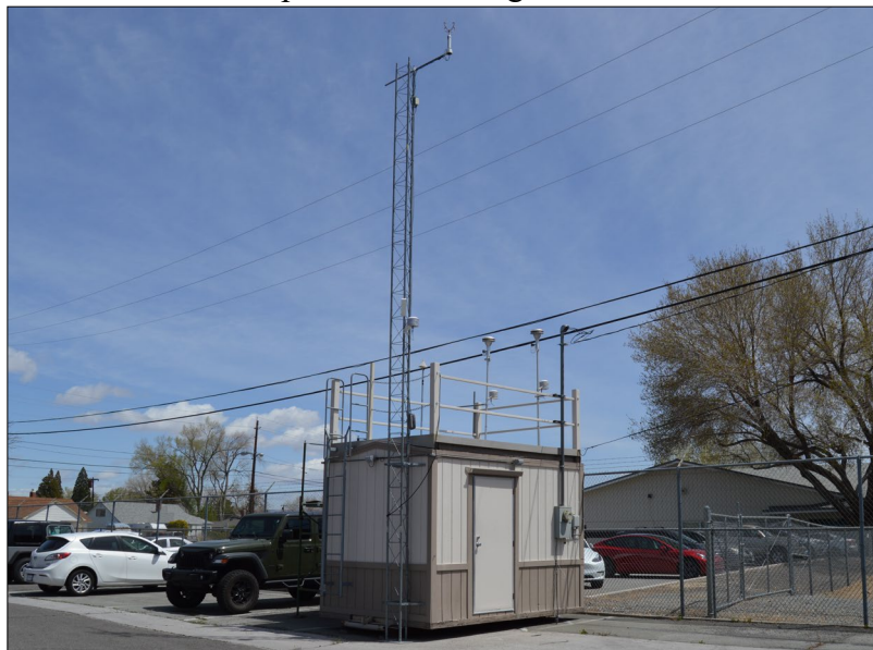
Figure 14 Sparks Monitoring Station
