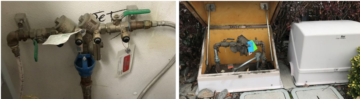
Figure 12: (Left) Typical installation of RPPA inside a food facility where piping is held 1" off wall using clear acrylic block and device has an air gap fitting installed on the drain line to ensure device is indirectly drained. (Right) RPPA installed in an outdoor hot box.
