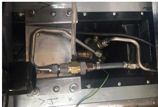
Figure 13: Dual check valve with intermediate atmospheric vent installed at beverage dispensing station.
