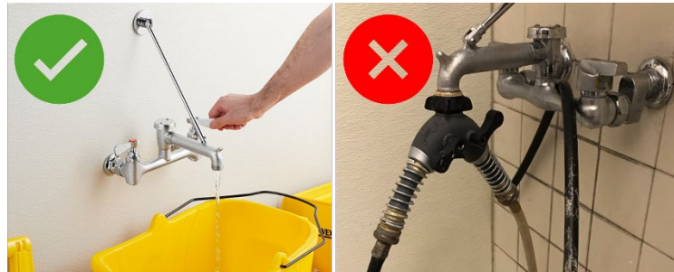
Figure 14: (Left) Properly installed atmospheric vacuum breaker on mop sink faucet. (Right) Prohibited y-valve connector installed on mop sink faucet that must be removed.
