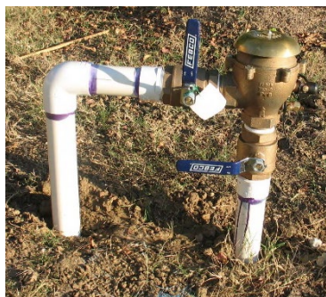
Figure 16: Pressure vacuum breaker installed on irrigation system.
