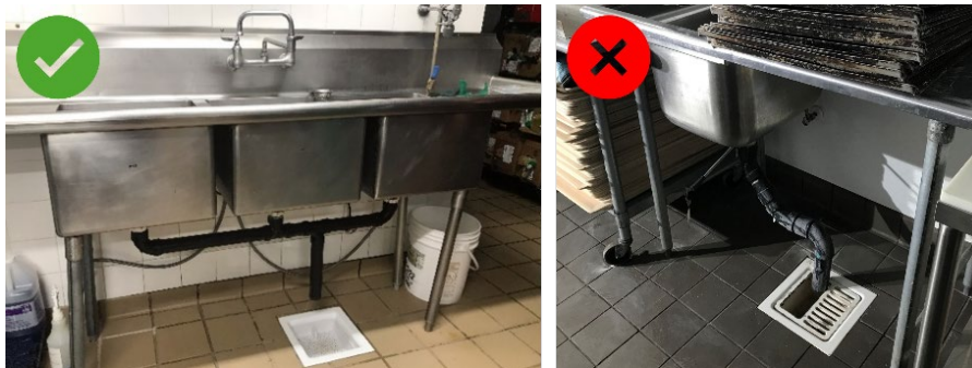
Figure 18: (Left) 3-compartment sink drain line properly air gapped to floor sink. (Right) Prep sink incorrectly plumbed with drain line below rim of floor sink.
